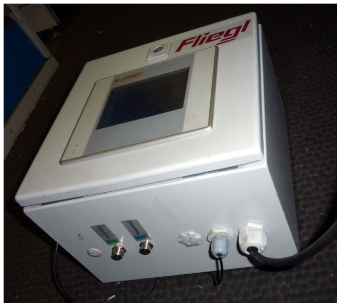
Fig. 2: Weighing machine switchgear cabinet - "DigiTouch Bio" as a weighing machine
